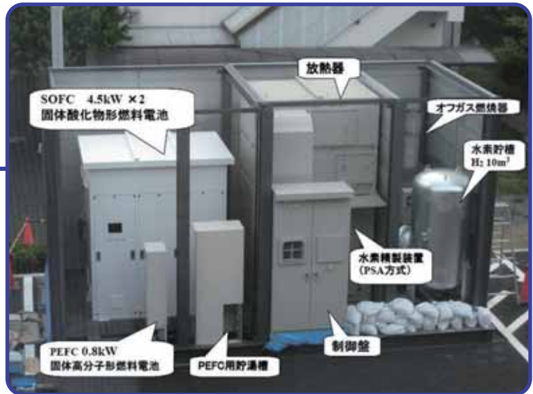
SOFC + PEFC Hybrid System (Tokyo Gas and Tokyo Institute of Technology)
